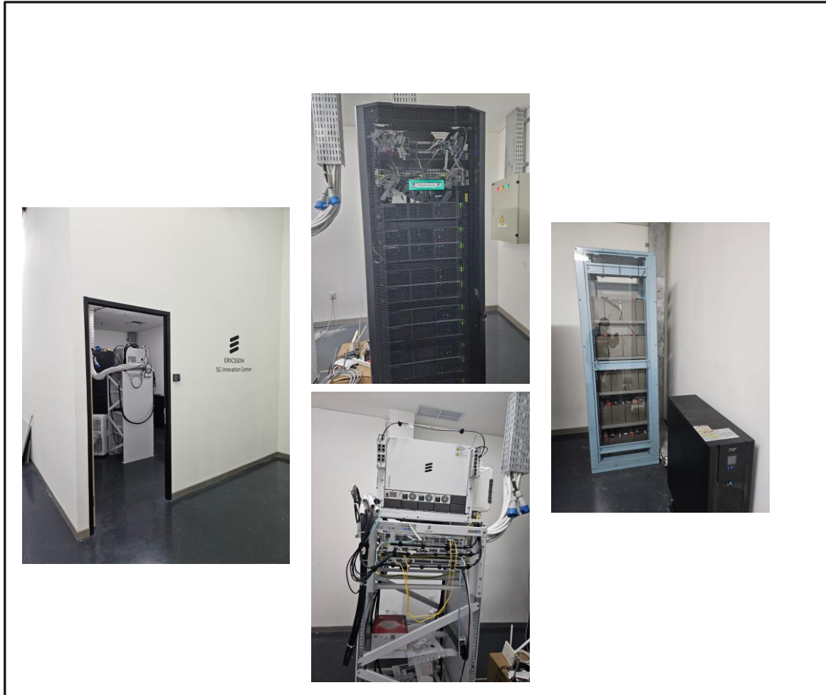
SA 5G Core Network at 2 nd Floor
